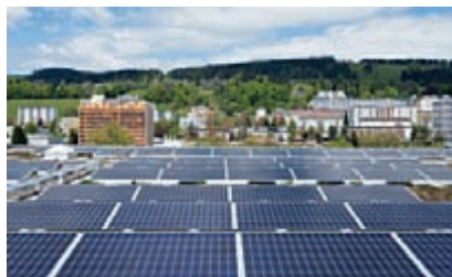
TAG Heuer's solar panels in La Chaux-de-Fonds.
