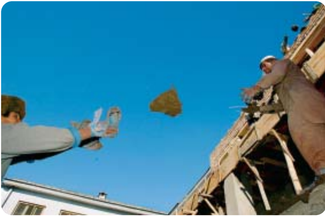
Afghan construction workers toss mud onto the roof being built at the Rabia Balkhi Women's Hospital in Kabul, Afghanistan.
